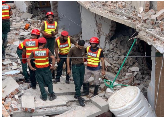
Building Collapse (Gujrat - 2021)
