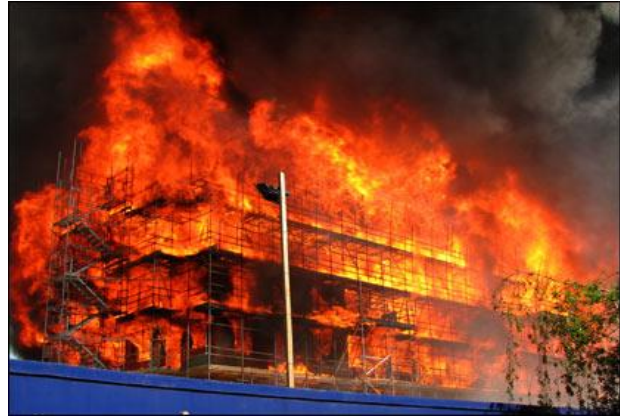
Fire incident at Lahori Gate, Lahore – Jan 2020
