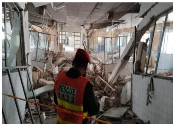
Building Collapse, Gujrat (2024)
