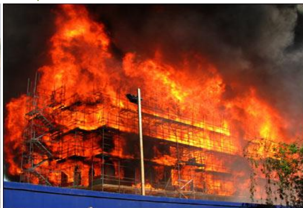
Fire incident at Lahori Gate, Lahore – Jan 2016
